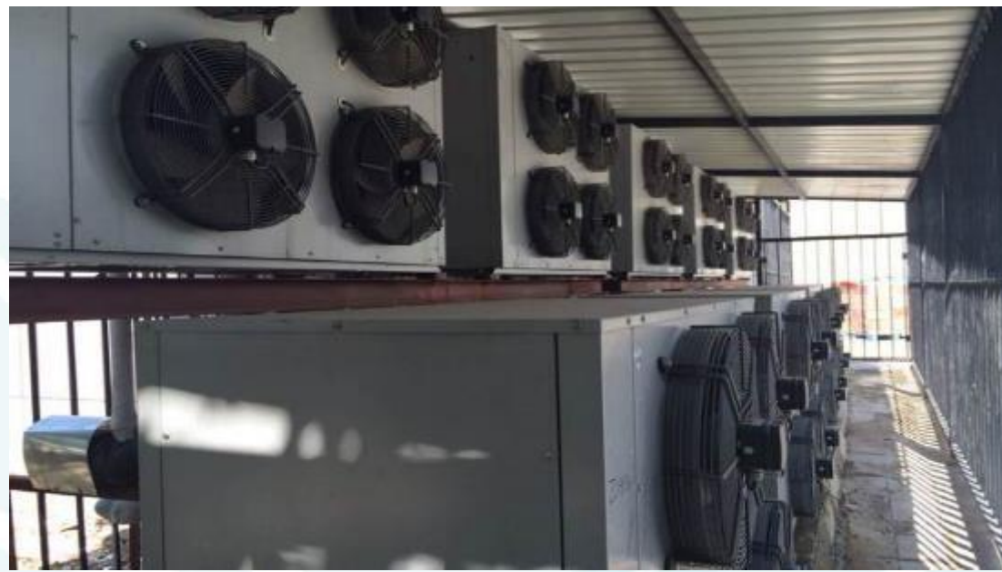
Air source heat pump project
